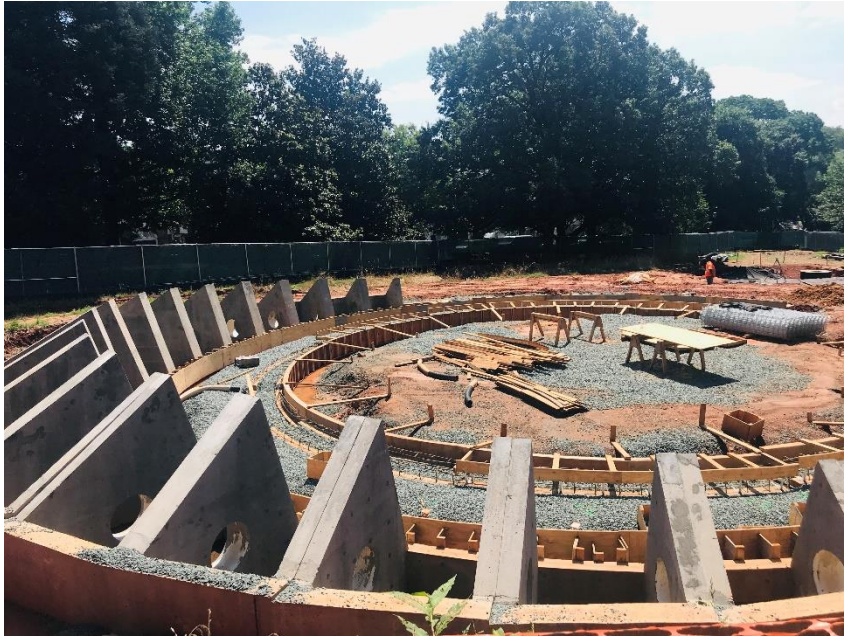
Fig. 2-3. Photos taken on site showing the current state of construction of the memorial.
